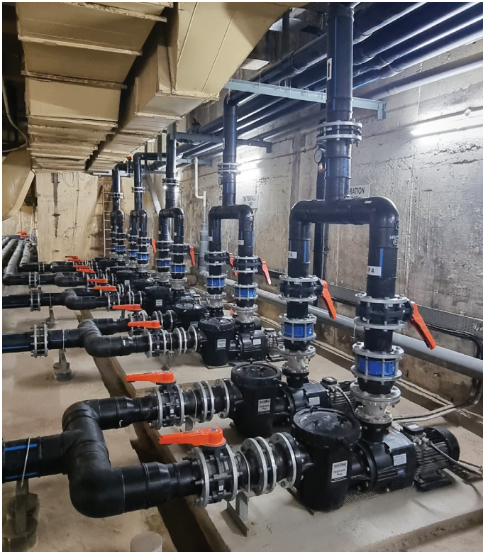
Waterco Series of High-Performance Pumps installed at Sunway Resort Hotel
