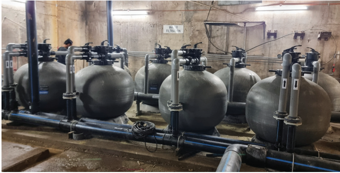
Waterco Micron Fibreglass Filters setup at Sunway Resort Hotel
