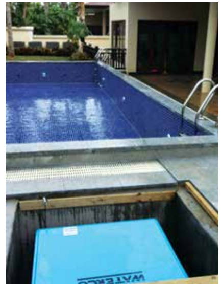
▲ Waterco supplied pumps including 5HP and 7HP Hydrostar commercial pumps and 3HP Hydrostorm Plus pumps, 6 Micron S1200 commercial fibreglass filters; and 26 WG600 all-in-one machines.
