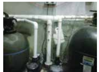
Ageing filtration system installed in 1992.
