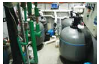
Four Micron SD750 fibreglass wound filters, with two high head Hydrostorm plus 200 pumps, and two MultiCyclone centrifugal pre-filters.
