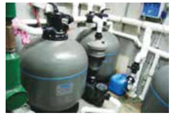
Each Hydrostorm plus 200 pump was plumbed to one MultiCyclone filter and the flow was split between two Micron SD750 filters.
