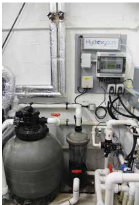
Hydroxypure system, a Waterco multicyclone centrifugal filter and a Certkin 24" Vision filter complete with glass media.
