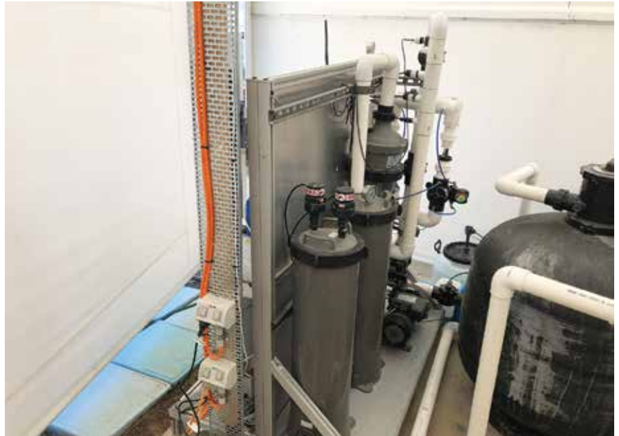
Somerset College's Hydroxypure commercial system.
