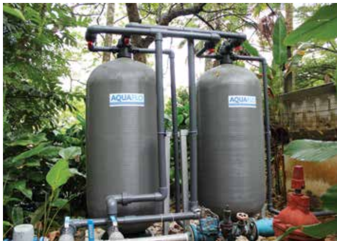
Aquaflo Top Mount Filters (AQ700X) setup at Tijani 2 North Condominium
