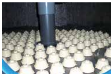
Nozzle Plate under drain system
