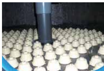
Nozzle Plate under drain system
